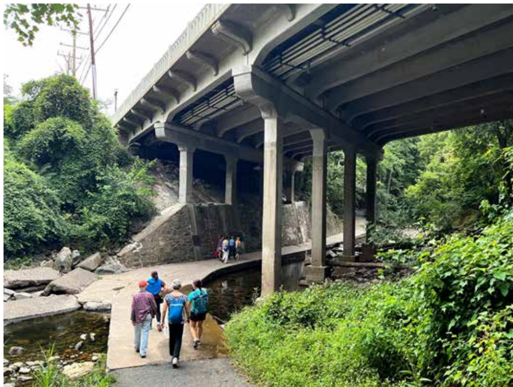
Trails Workgroup site visit on the W&OD trail, observing the eroded banks of the stream where the paved connector trails were built.
